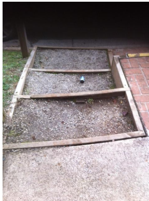
Steps - an accident waiting to happen
